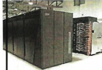
The Fermi BG/Q system installed at CINECA.
